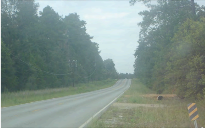
Fault line scarp on LA Highway 441 approximately one half mile south of Interstate 12. View to the North. (Used by permission.)
