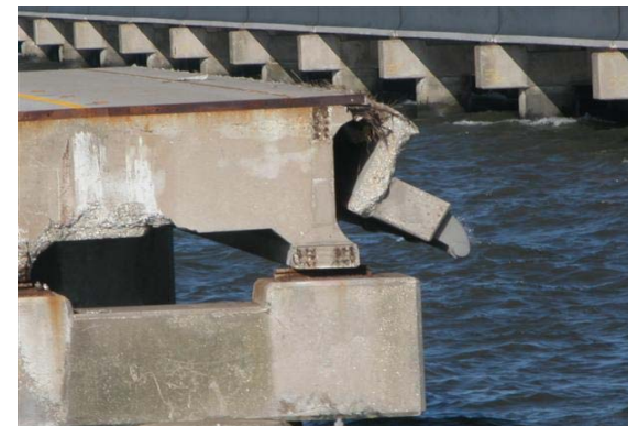
Damage to I-10 (twin span near New Orleans, LA)
